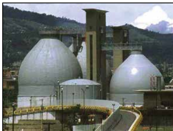
Typical industrial wastewater digester
