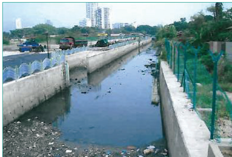
Fig. 2 Additional pictures of the pond and drainage system
