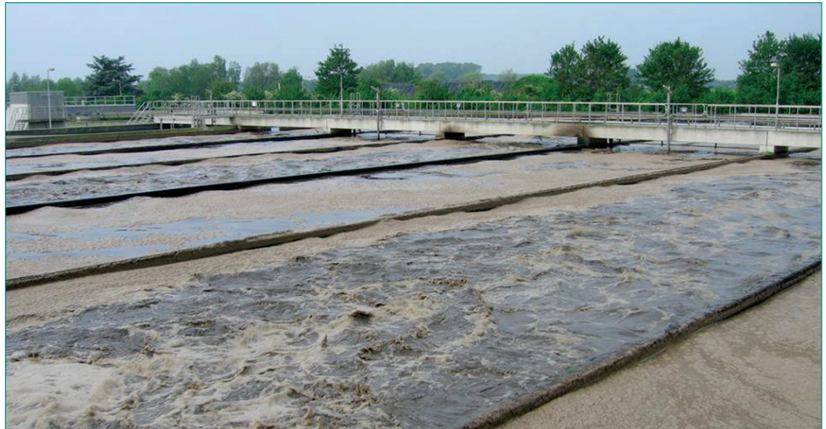
Fig. 1: This picture shows the parallel aerated basins side by side. Since these trains have segregated recycle lines they can be treated separately and the sludge from each train can be evaluated and compared.
