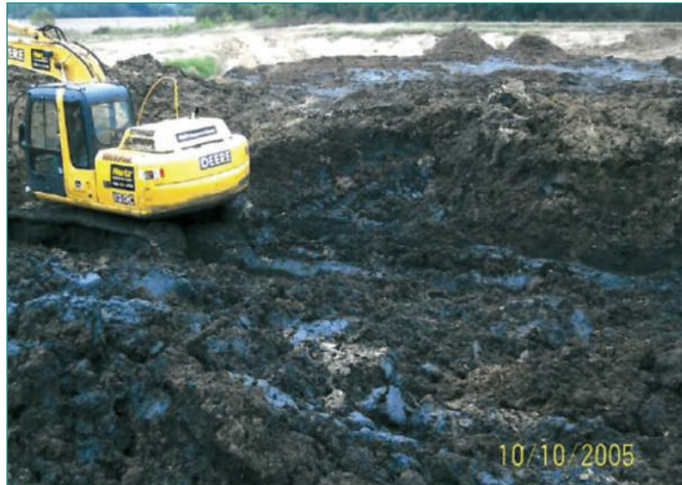
Fig 2: Excavation to ready the site for land farming shows the extent of contamination.
